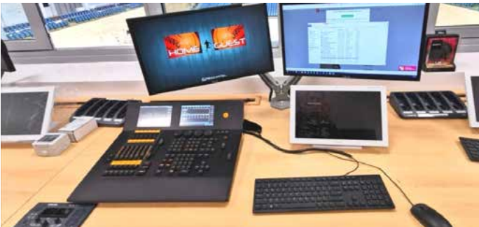
The Control Room at the Mezzanine floor, with all its AV gear (with a see-through window to the two halls).
