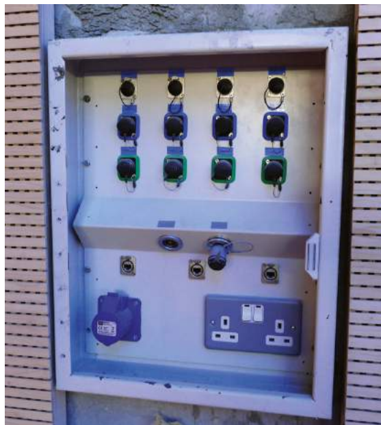
AV control is achievable from any location in the field via tielines in distributed broadcast boxes
